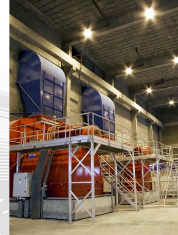
Ventilation in tunnel
